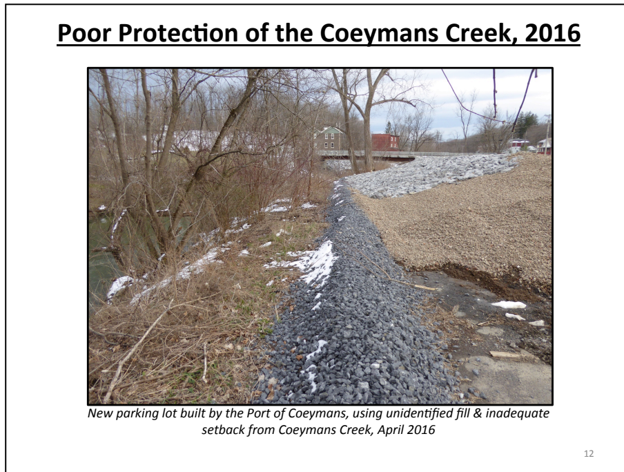
Figure 10: In violation of laws requiring a 50-foot setback, this parking lot was constructed with unidentified fill from the Port of Coeymans
