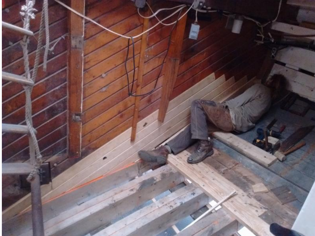
The bulkhead (the wall on a ship) between the engine room and captain's cabin being rebuilt.
