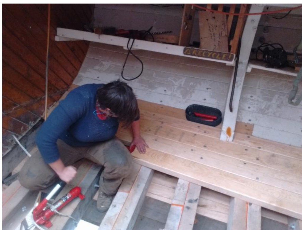
Emily is pushing a ceiling plank into place. This one had to go underneath the bulkhead between the hold and the focsle, so a lot of force was needed to get it in place, thus the porta power.
