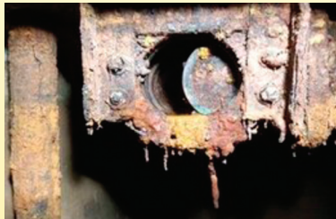
Pipe corrosion leading to a major leak in the IP-1 fuel pool, which caused significant contamination of ground water under the plant.
