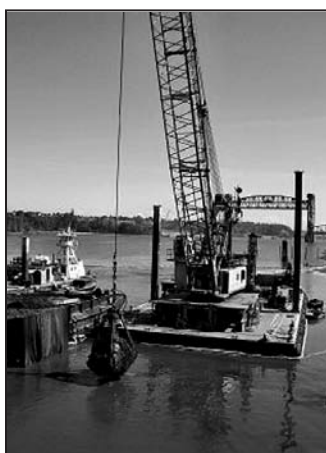
An example of a clamshell dredge that will be used to remove PCB-contaminated sediment from a series of “hotspots” in the river bottom located in a 40-mile stretch of the Upper Hudson.
